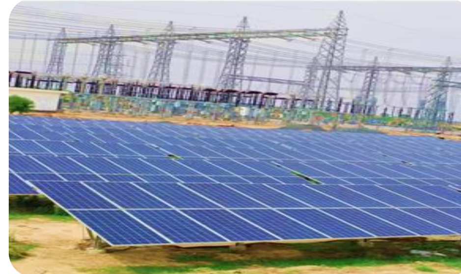
ATL moving progressively towards goal of 100% auxiliary power through solar PV installation at substations
