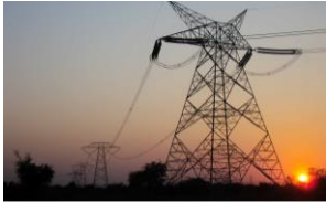
Longest Private HVDC Line in Asia
