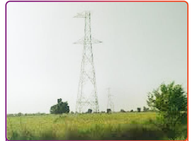
765kV Ghatampur TPS-Agra SC line
