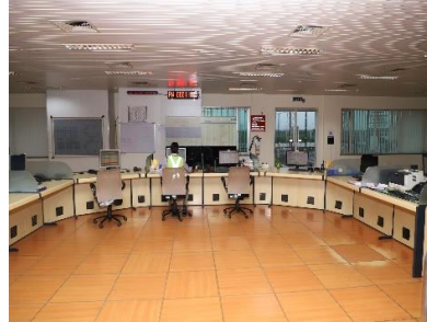
Remote operation of substations (ENOC)
