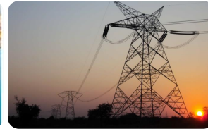
Longest Private HVDC Line in Asia
