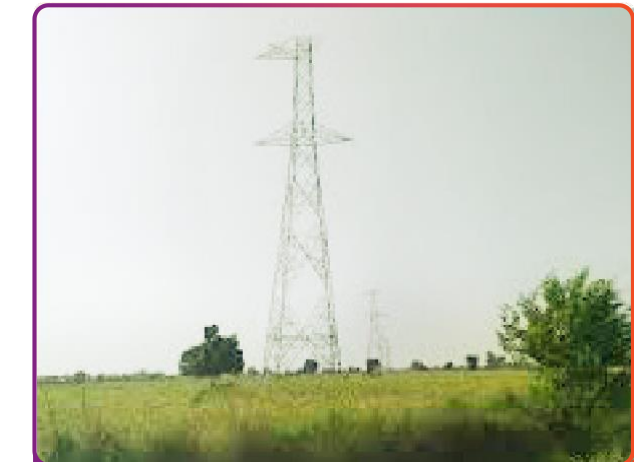
765kV Ghatampur TPS-Agra SC line
