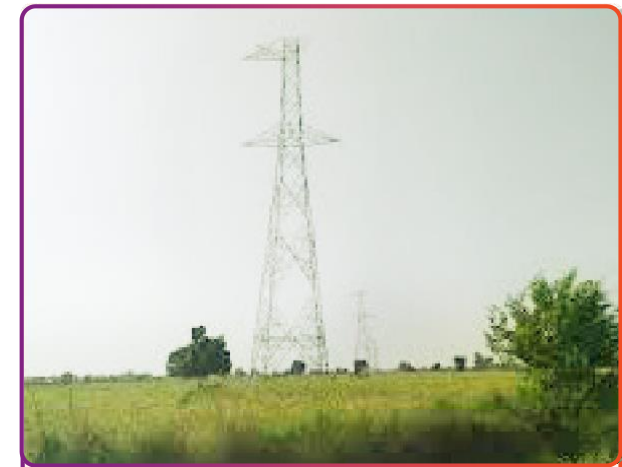
765kV Ghatampur TPS-Agra SC line
