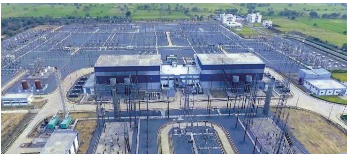
± 500 kV HVDC Mohindergarh Substation
