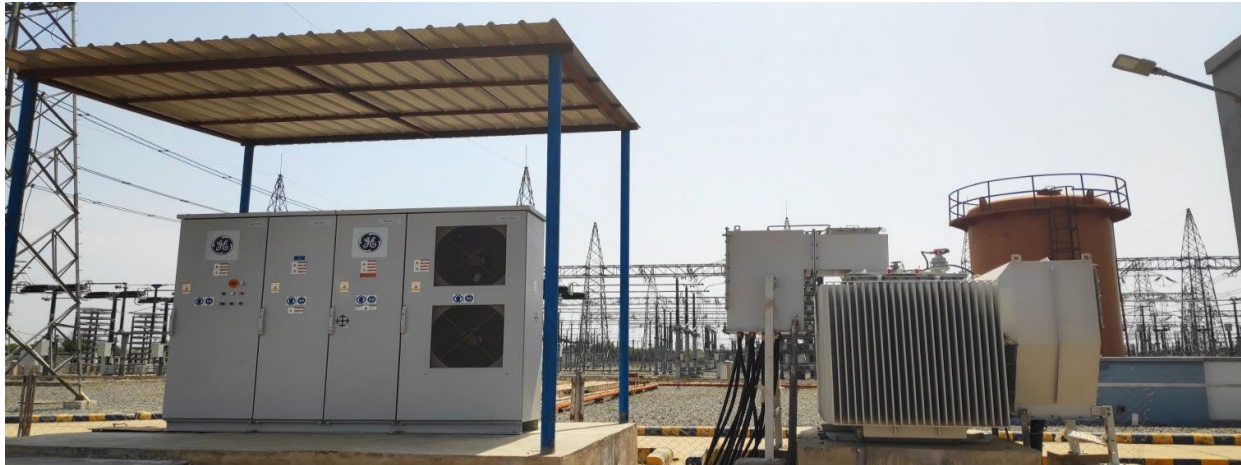
APFC Panel and Transformer
